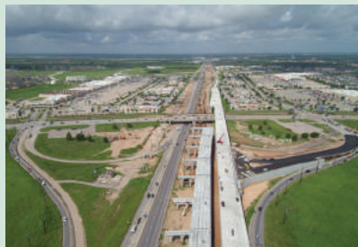
August 2017: I-69 southbound at FM 762, a year later, the new exit ramp nearly ready.
